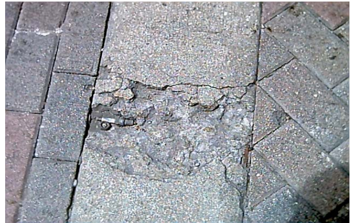
Damaged Crosswalk on Northwood Road
