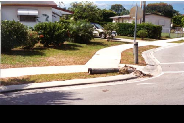
Damaged Bollard at Golf and 7 th Street
